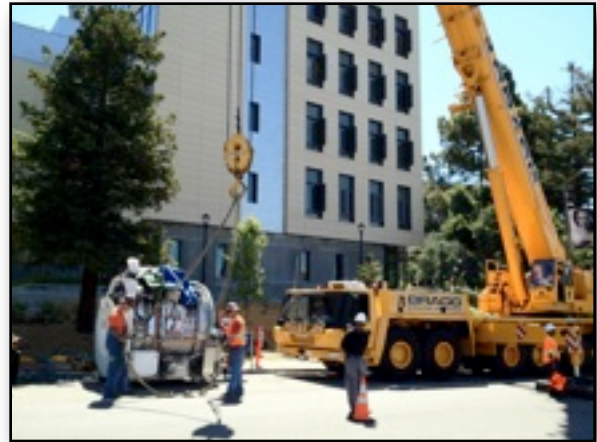
MRI machinery being installed at the Li Ka Shing Center. Photo by Dr. Ben Inglis.
